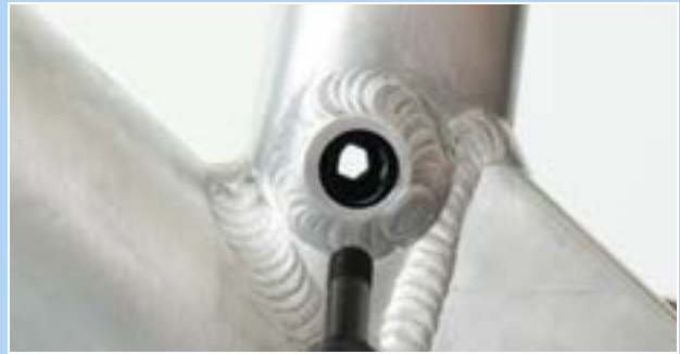
Figure 210: Hole in the Postpin interface
